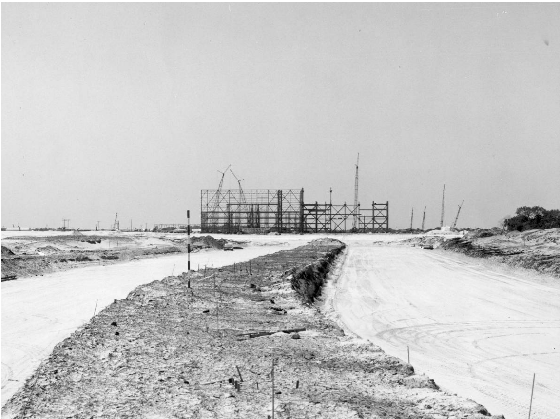
Figure A-5. View of Crawlerway construction, near VAB, March 30, 1964. Source: John F. Kennedy Space Center Archives, KSC-64-2873.
