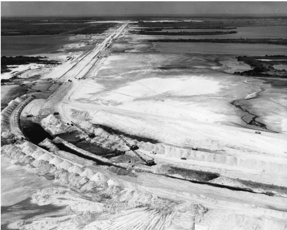
Figure A-6. View of Crawlerway construction, April 7, 1964. Source: John F. Kennedy Space Center Archives, KSC-64C-994.
