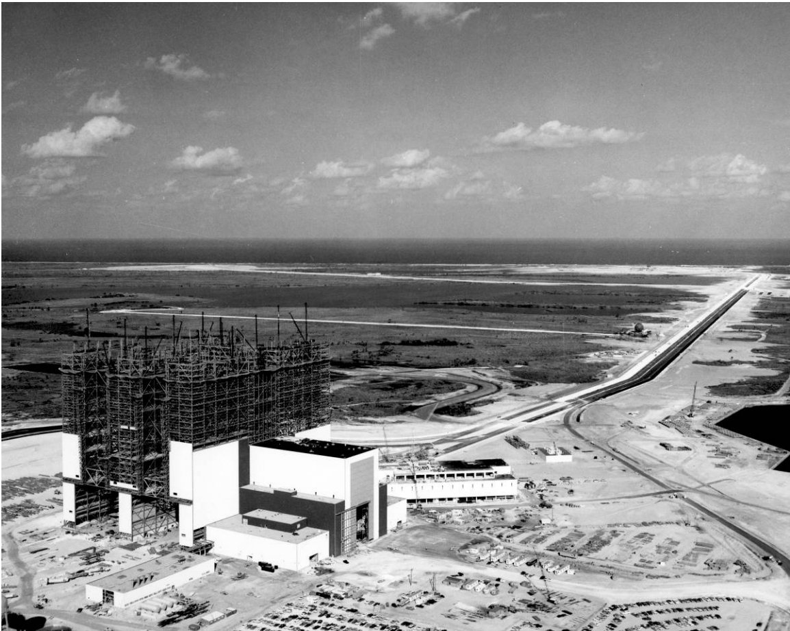
Figure A-8. Aerial view of LC 39 construction, showing VAB in foreground and Crawlerway in background and at right, January 28, 1965.
