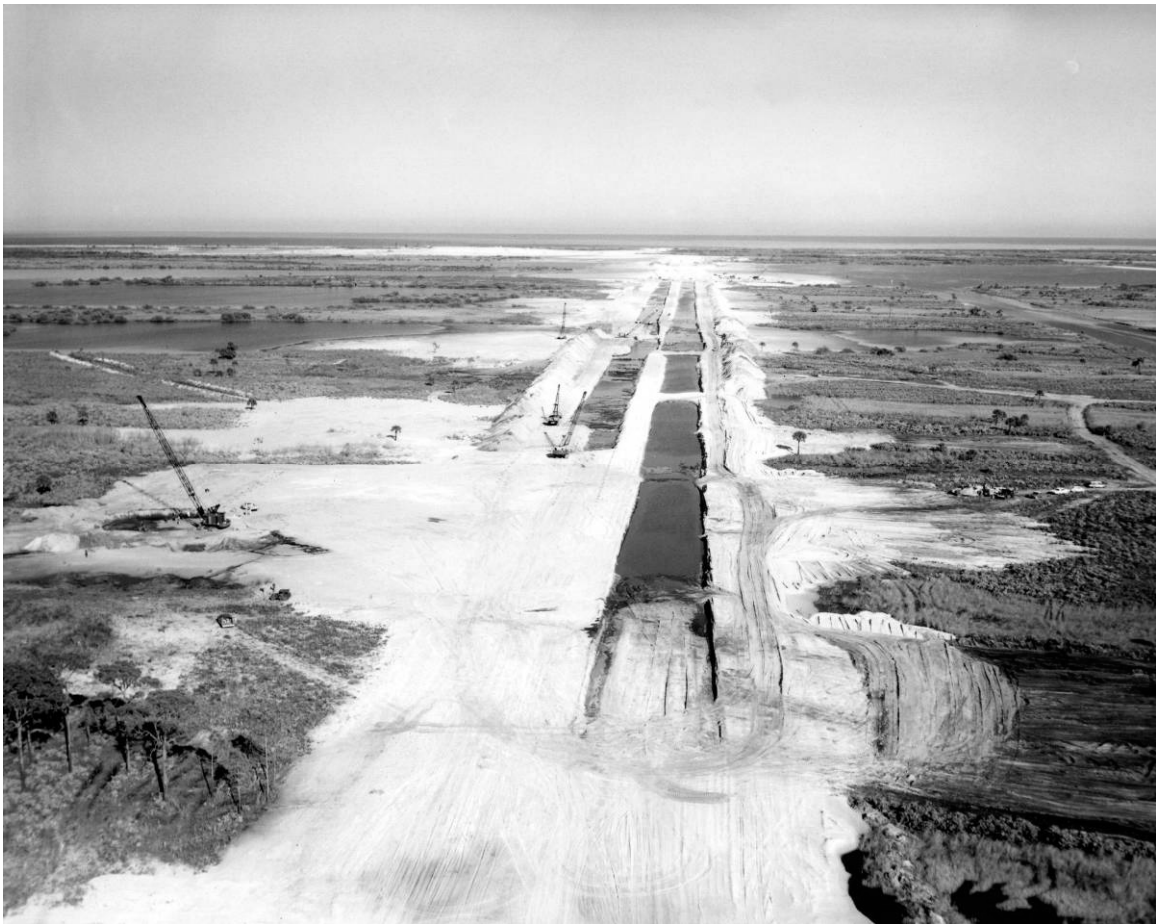
Figure A-4. View of Crawlerway construction, December 26, 1963. Source: John F. Kennedy Space Center Archives, KSC-64C-7.
