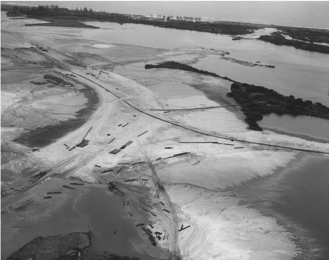
Figure A-3. View of Crawlerway construction, showing hydraulic fill, April 30, 1963. Source: John F. Kennedy Space Center Archives, LOC-63-4457.
