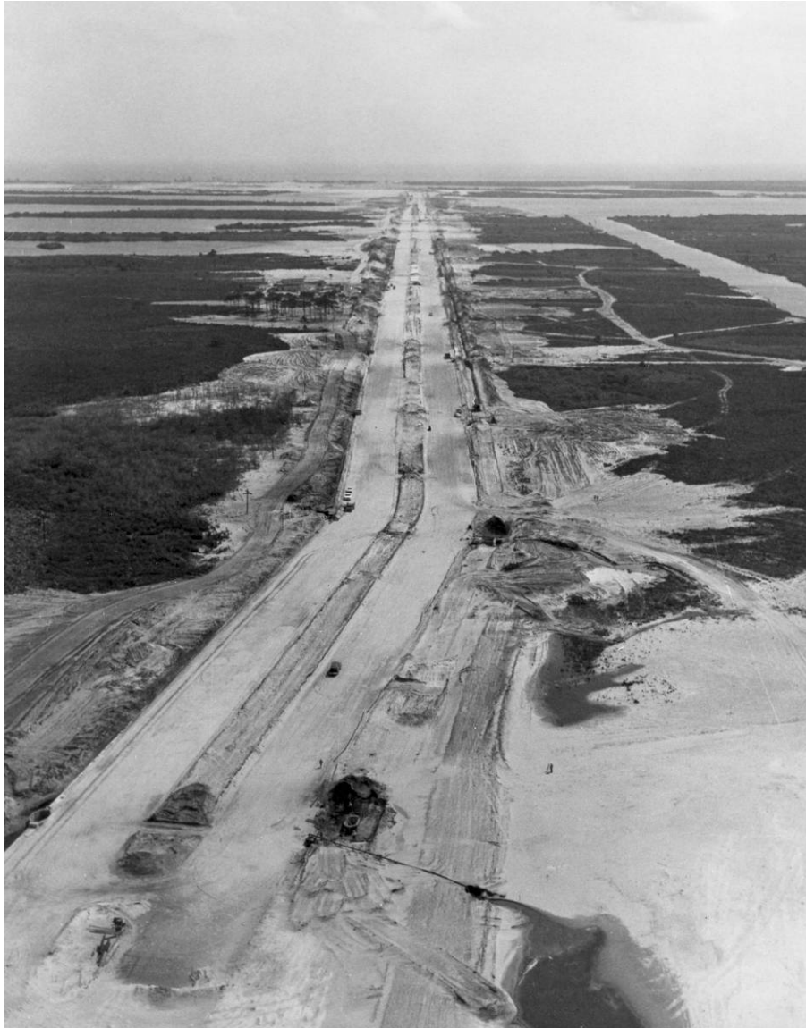
Figure A-7. View of Crawlerway construction, April 7, 1964. Source: John F. Kennedy Space Center, KSC-64C-1008.
