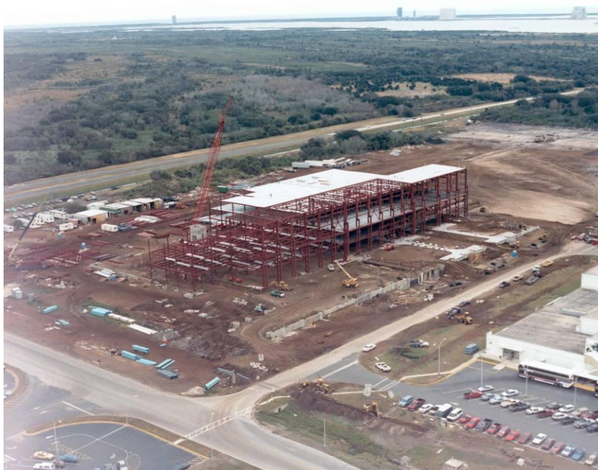
Photo 11. Aerial view showing construction of SSPF, January 1992, facing northeast. (KSC Archives, KSC-392C-326.02).
