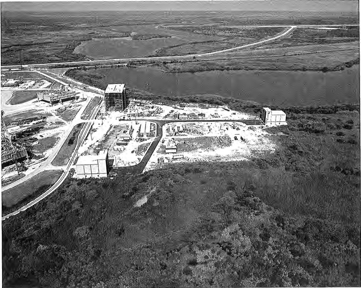
Aerial View of RPSF Complex Under Construction, View to West, July 5, 1983 (Courtesy of Kennedy Space Center, Negative 108- KSC-383C-2203-40).
