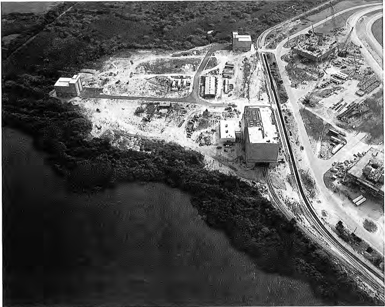
Aerial View of RPSF Complex Under Construction, View to East, October 4, 1983 (Courtesy of Kennedy Space Center, Negative 116- KSC-383C-3561-100).
