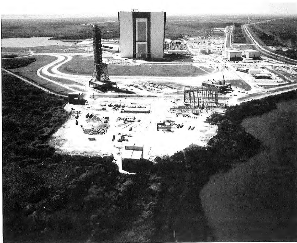
Aerial View of RPSF Complex Under Construction, Showing RPSF Steel Frame, View to South, April 21, 1983 (Courtesy of Kennedy Space Center, Negative 108-KSC-383C-1085-90).
