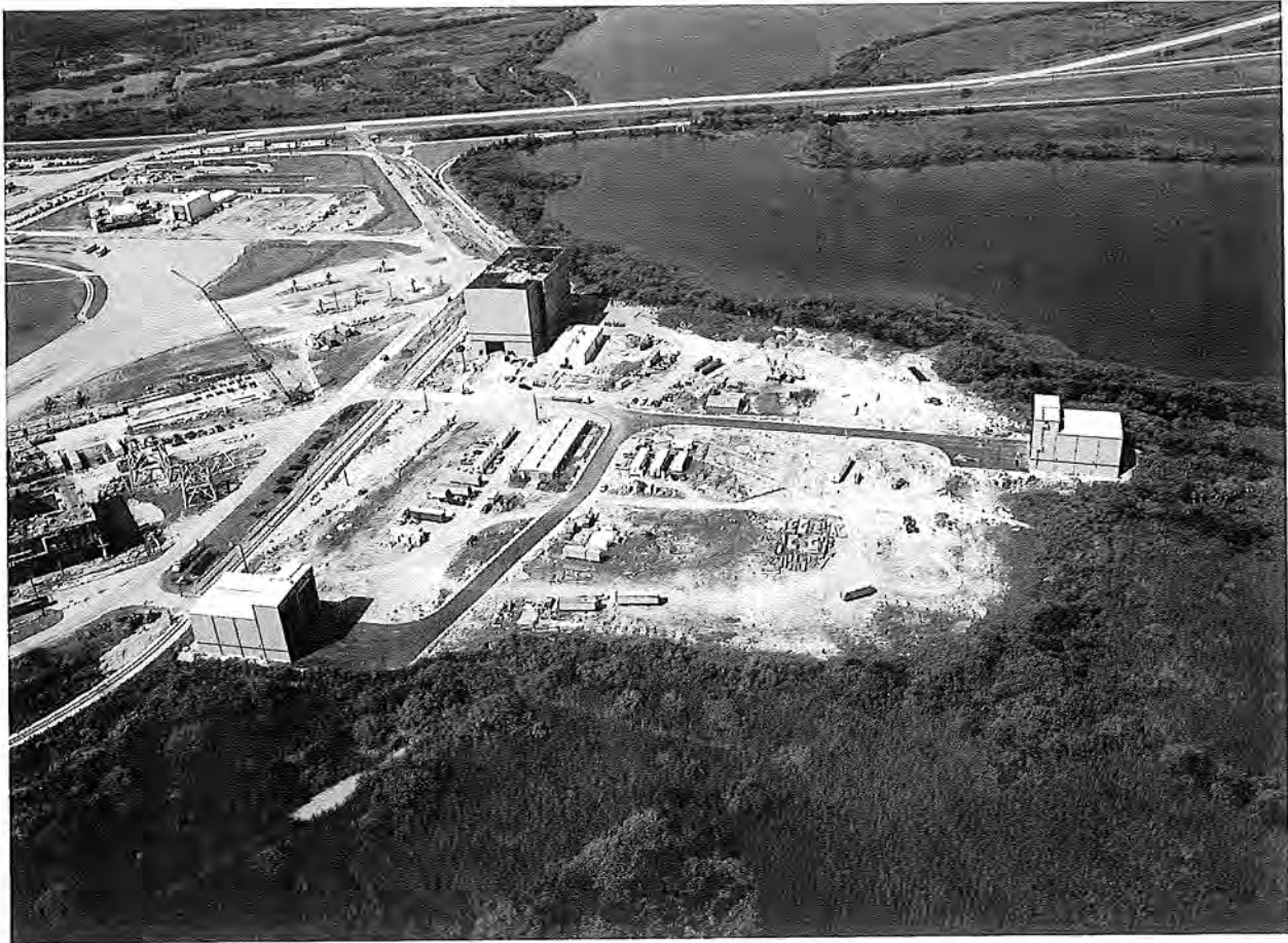
Aerial View of RPSF Complex Under Construction, View to West-Southwest, September 1, 1983 (Courtesy of Kennedy Space Center, Negative 116-KSC-383C-3090-30).
