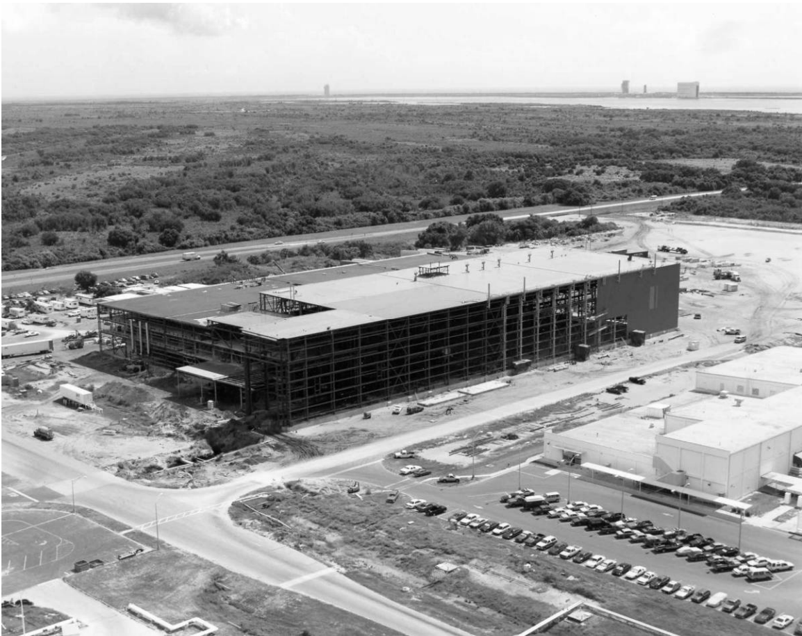
Figure A-4. View of SSPF, showing construction progress, camera facing northeast, July 13, 1992.
