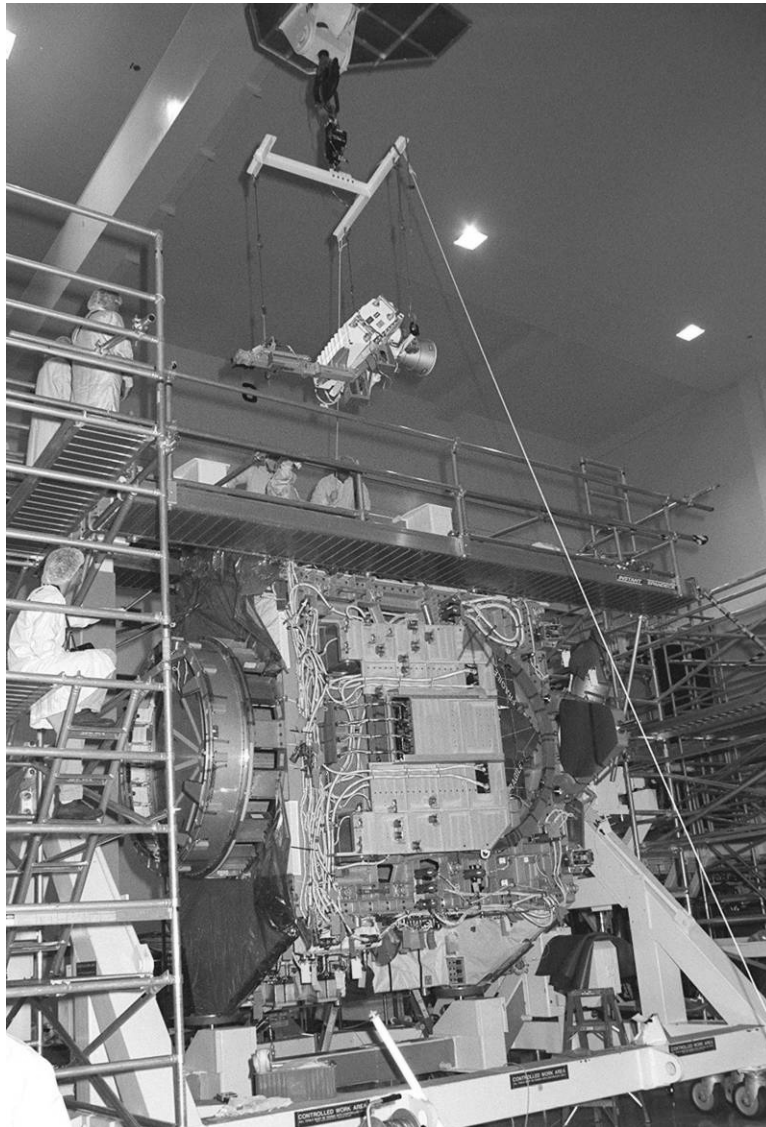
Figure A-14. An S-band Antenna Support Assembly being installed on the Z1 Truss, camera facing northeast, June 6, 2000.
