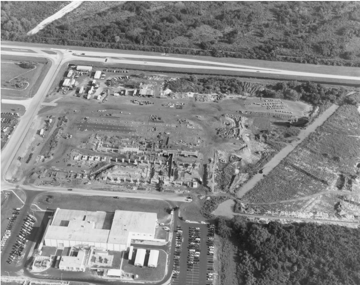
Figure A-1. View of SSPF site during initial construction efforts, camera facing north, September 27, 1991.
