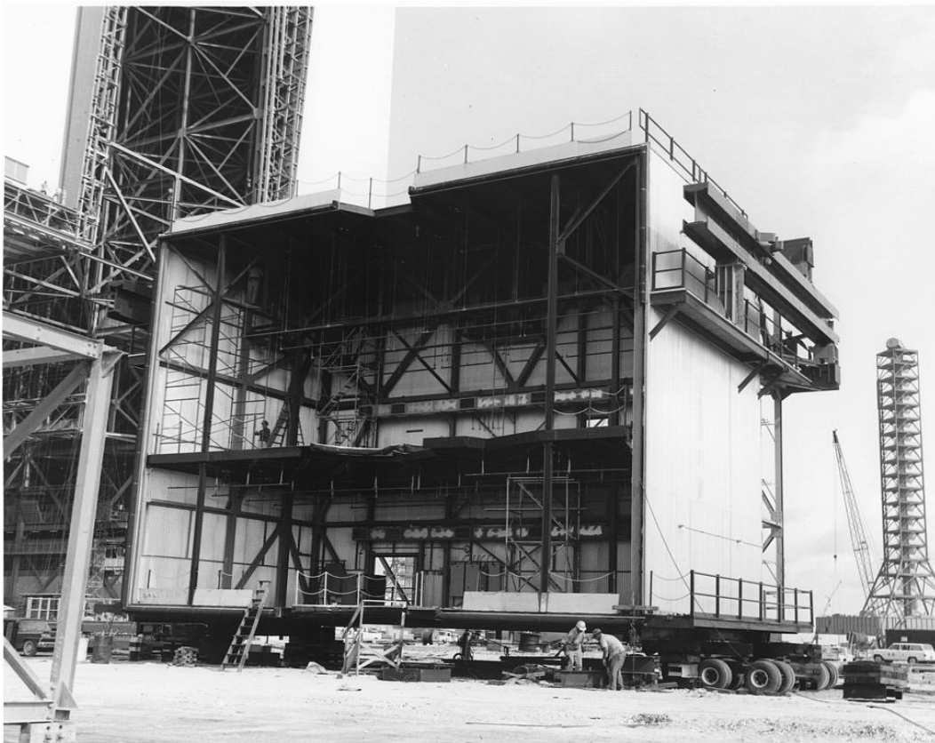
Photo A-5. Construction of Vehicle Assembly Building, 9 August 1965. Source: John F. Kennedy Space Center, KSC-65C-5327, accessed via NIX at http://nix.nasa.gov/ .
