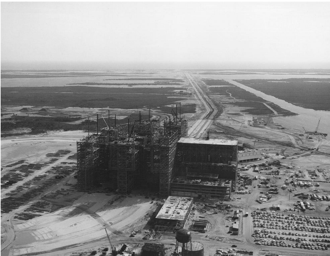
Photo A-3. Early phase of steel construction of Vehicle Assembly Building, 13 October 1964. Source: John F. Kennedy Space Center, KSC-64C-4000, accessed via NIX at http://nix.nasa.gov/ .
