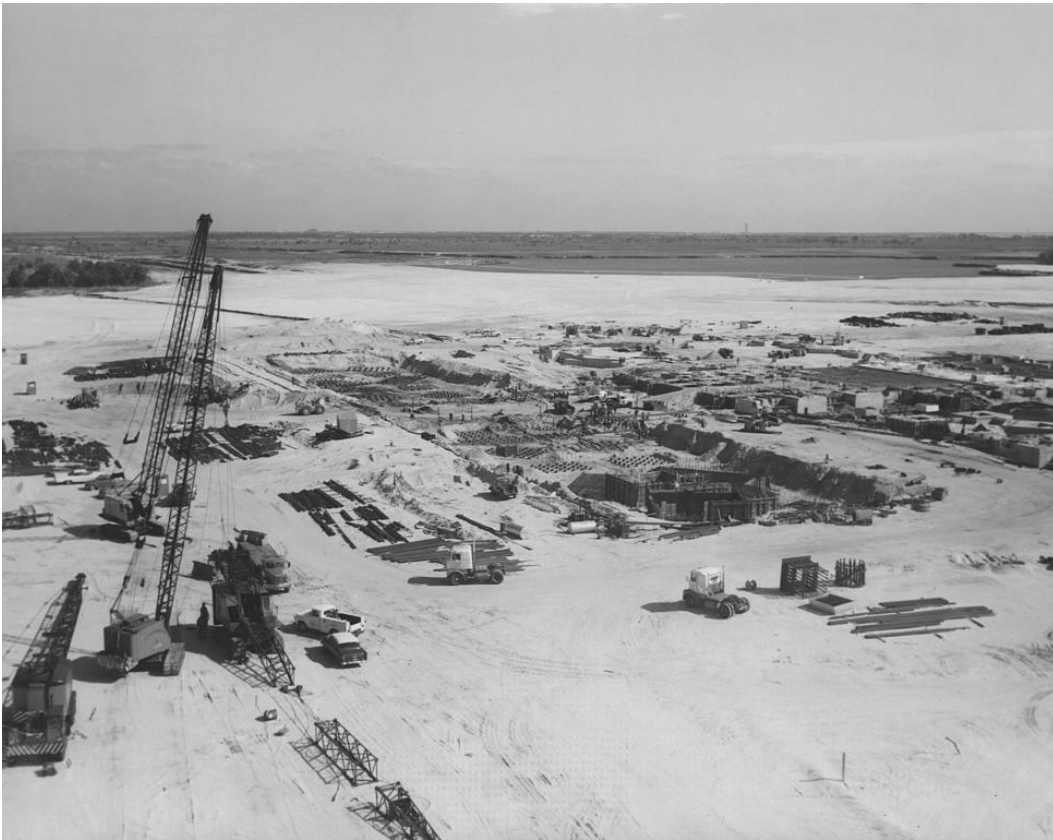
Photo A-2. Construction of Vehicle Assembly Building foundation, 14 January 1964. Source: John F. Kennedy Space Center, KSC-64C-0276, accessed via NASA Image Exchange (NIX) at http://nix.nasa.gov/ .
