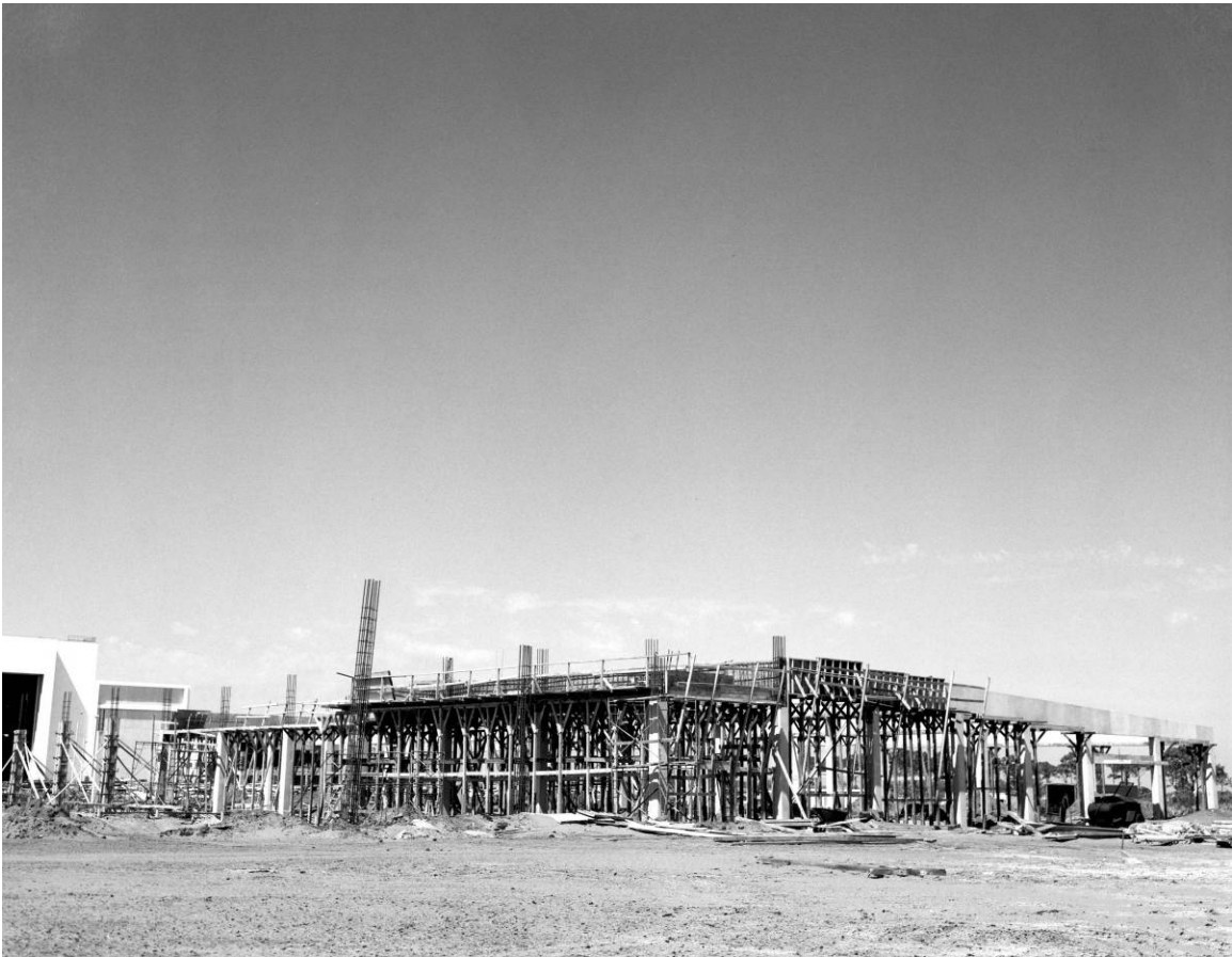
Figure A-2. Construction of the Flight Crew Training Building, March 9, 1965. Source: John F. Kennedy Space Center Archives, 100-KSC-65-5371.
