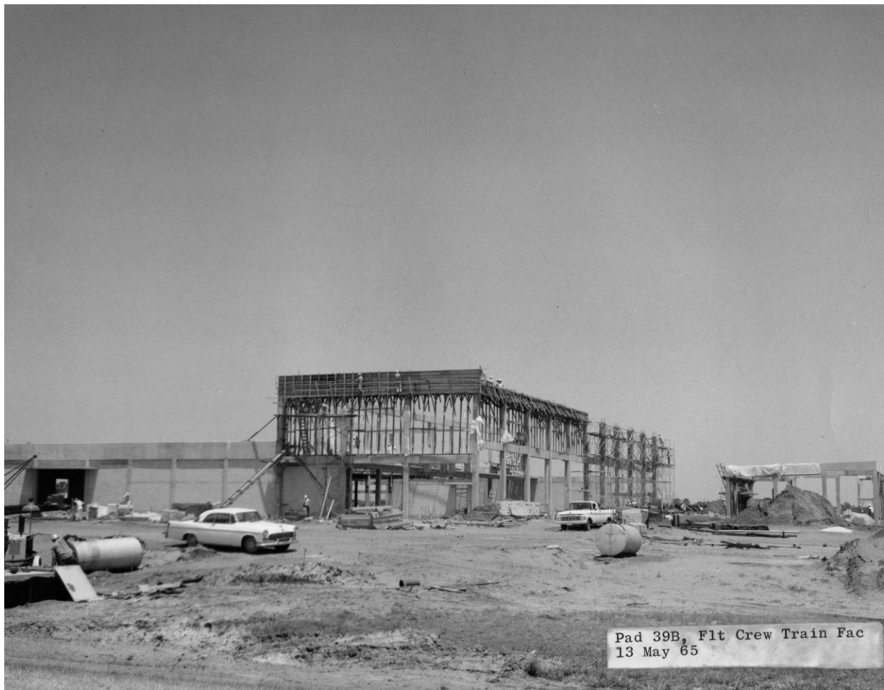
Figure A-3. Construction of the Flight Crew Training Building, May 13, 1965. Source: John F. Kennedy Space Center Archives, 100-KSC-65-9379.
