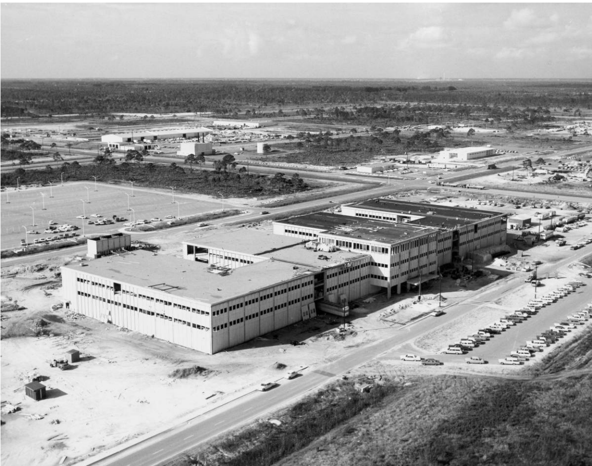
Figure A-11. View showing Phase I construction of the Headquarters Building, facing southwest, October 13, 1964.
