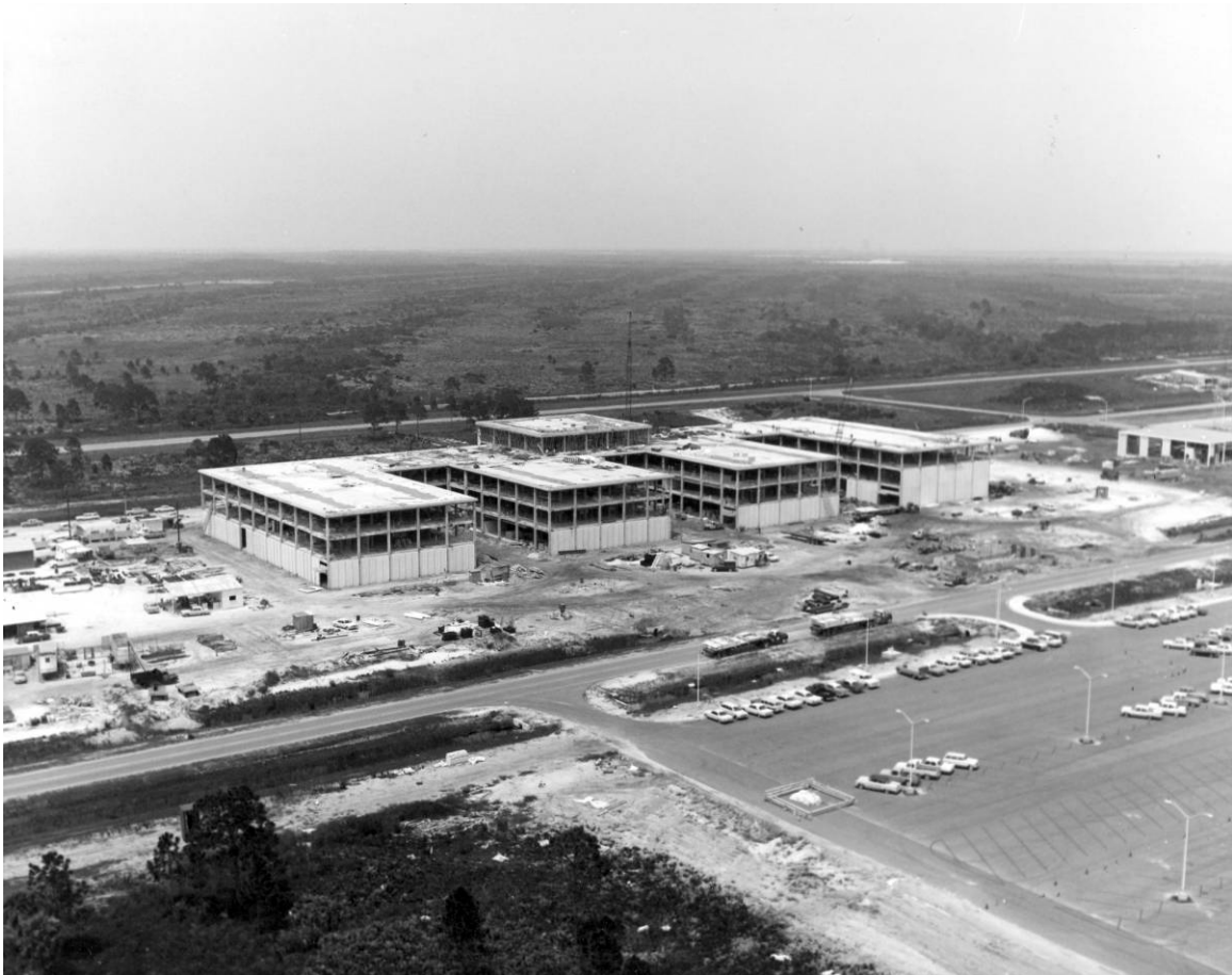
Figure A-10. View showing Phase I construction of the Headquarters Building, facing northeast, August 6, 1964.
