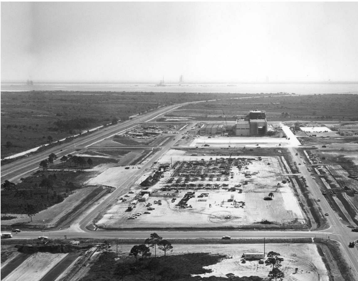
Figure A-9. View showing site preparations for the construction of the Headquarters Building, facing east, March 5, 1964.
