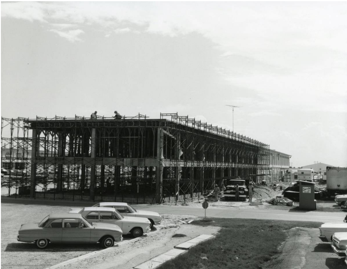
Figure A-5. View of the construction of the North Wing addition to the E&O Building, April 2, 1963.
