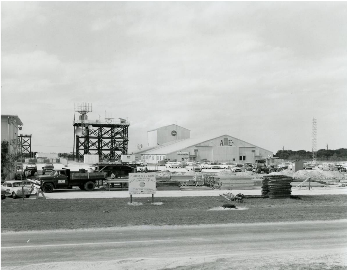
Figure A-4. Construction materials for the North Wing addition to the E&O Building, January 25, 1963.
