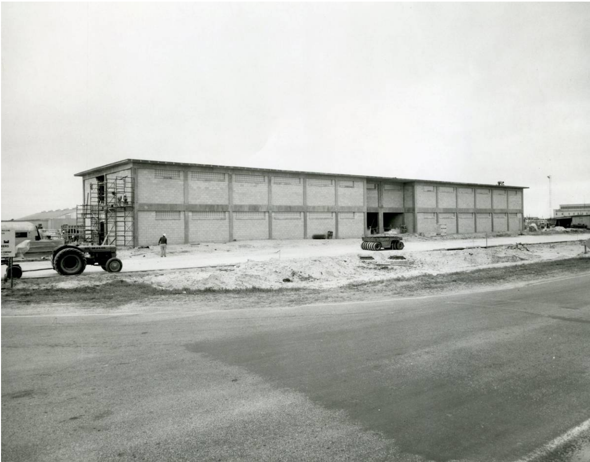
Figure A-2. Construction work on the E&O Building, February 1, 1961. Source: John F. Kennedy Space Center Archives, LOD-61-948.
