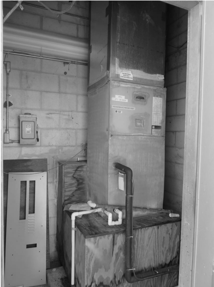
Figure A-4. Mechanical Room of the Solar Array Test Building, facing southeast, August 26, 2014.
