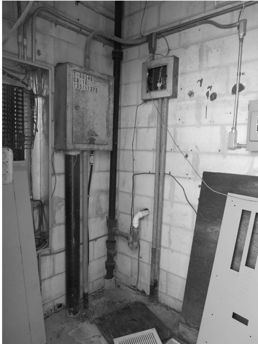
Figure A-5. Mechanical Room of the Solar Array Test Building, facing northeast, August 26, 2014.
