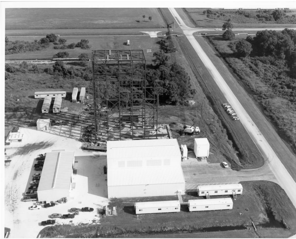
Figure A-2. View of CRF, showing the assembly of the steel skeleton, camera facing north, October 4, 1991.
