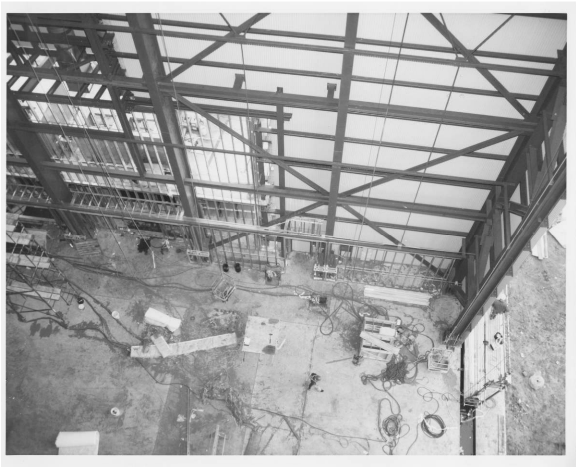
Figure A-5. Interior view of CRF during construction, camera facing north, January 24, 1992. Source: John F. Kennedy Space Center Archives, KSC-392C-342_08.
