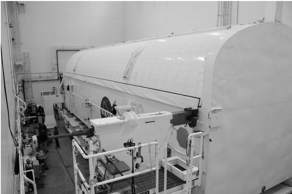
Figure A-9. Detail view showing a U-saddle (near right of photo), April 13, 2010. Source: Penny Rogo Bailes.
