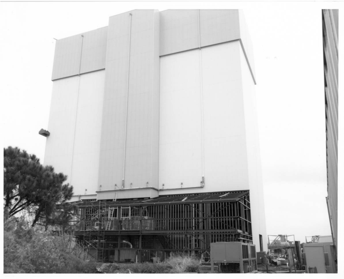
Figure A-3. View of CRF, showing completed exterior walls and steel skeleton of the mechanical building to the north, camera facing southeast, January 24, 1992.
