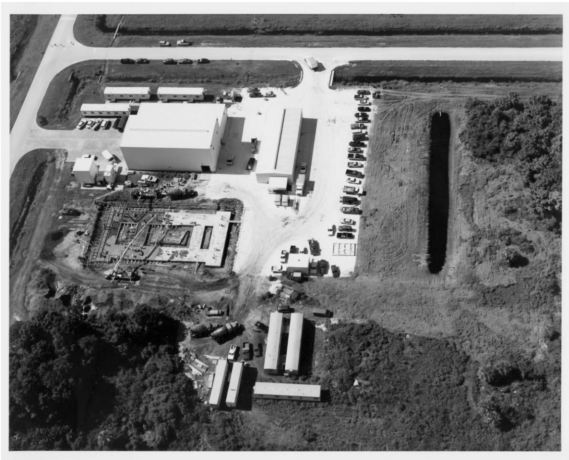
Figure A-1. View of CRF under construction, showing foundations, camera facing south, August 6, 1991.
