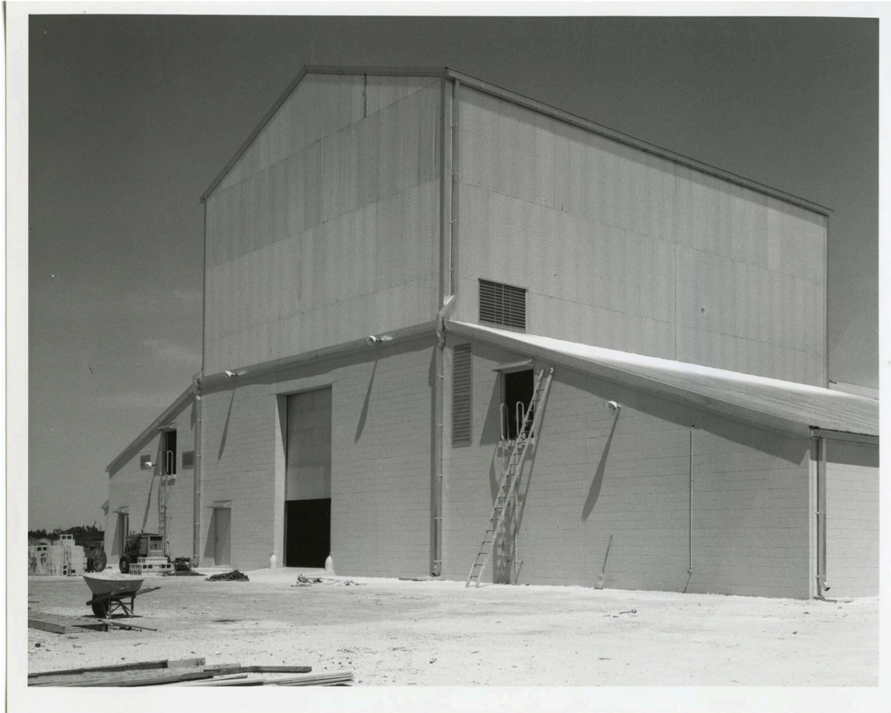
Figure 8. Hangar AE high bay under construction, 1961. (Courtesy of Kennedy Space Center Archives, Image LOD-61-4343).
