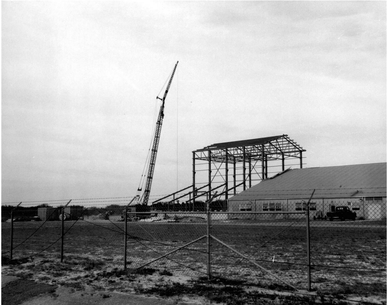
Figure 6. View of Hangar AE high bay under construction, 1961. (Courtesy of Kennedy Space Center Archives, Image LOD-61-2146).
