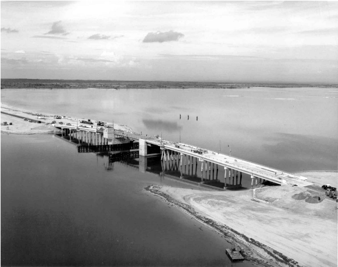
Figure B-6. Construction of the Banana River Bridge, facing northwest, January 8, 1964. Source: John F. Kennedy Space Center Archives, KSC-64-400.
