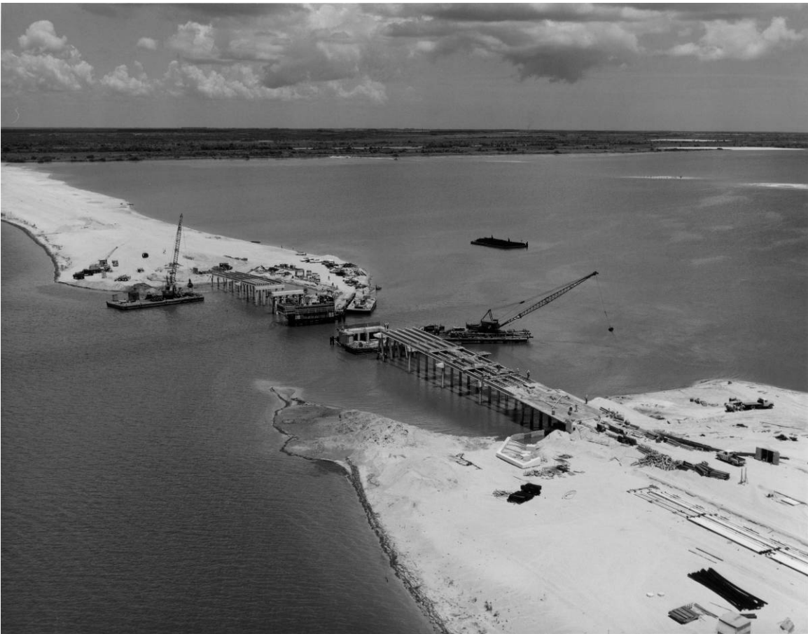
Figure B-2. Construction of the Banana River Bridge, facing northwest, June 30, 1963. Source: John F. Kennedy Space Center Archives, LOC-63-7706.
