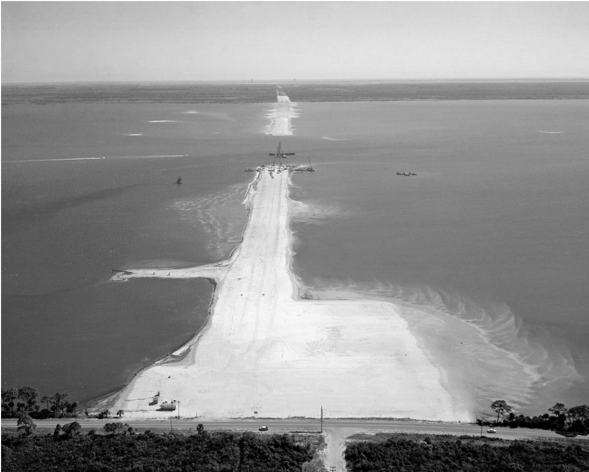
Figure B-8. Hydraulic fill and early construction of the Indian River Bridge, facing east, October 30, 1963.
