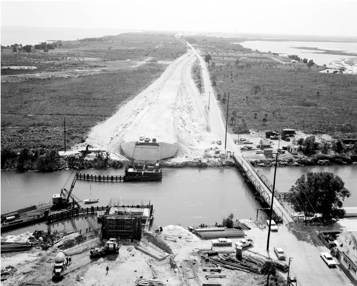
Figure A-2. Construction of the Haulover Canal Bridge (old wooden bridge to right), camera facing southeast, March 11, 1965.
