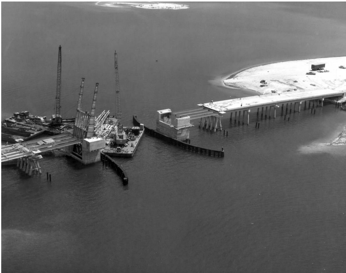
Figure B-4. Construction of the Banana River Bridge, facing northeast, September 5, 1963. Source: John F. Kennedy Space Center Archives, LOC-63-8790.
