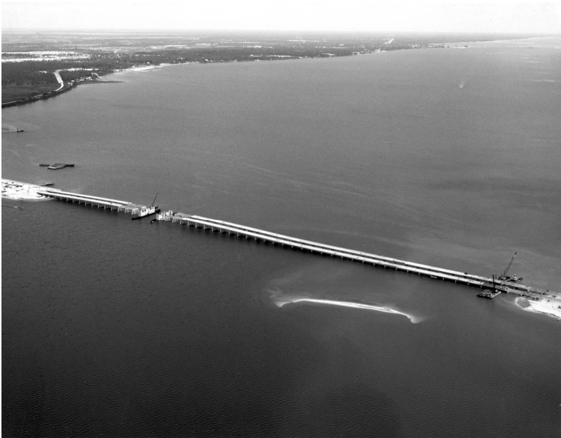
Figure B-10. Construction of the Indian River Bridge, facing northwest, May 11, 1964. Source: John F. Kennedy Space Center Archives, KSC-64-3714.
