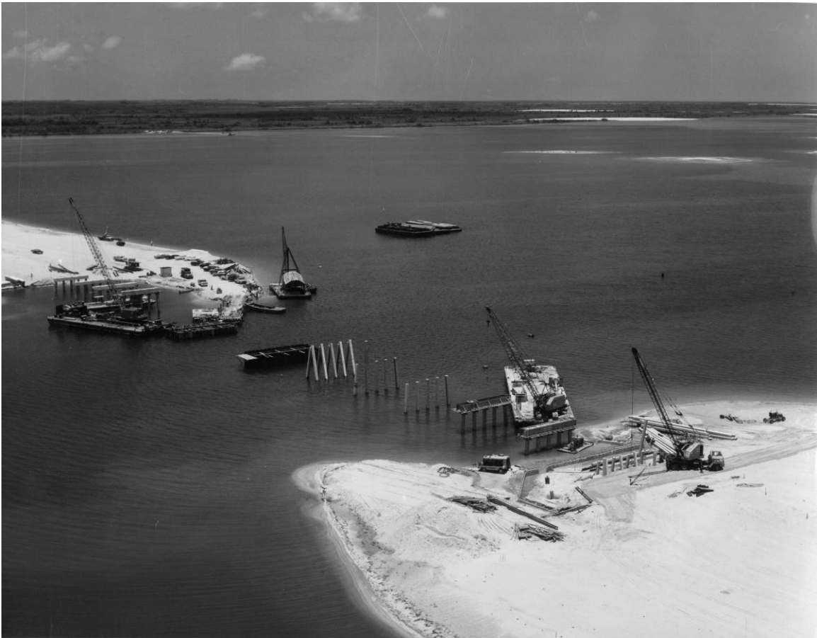
Figure B-1. Early construction of the Banana River Bridge, facing northwest, June 4, 1963. Source: John F. Kennedy Space Center Archives, LOC-63-5649.
