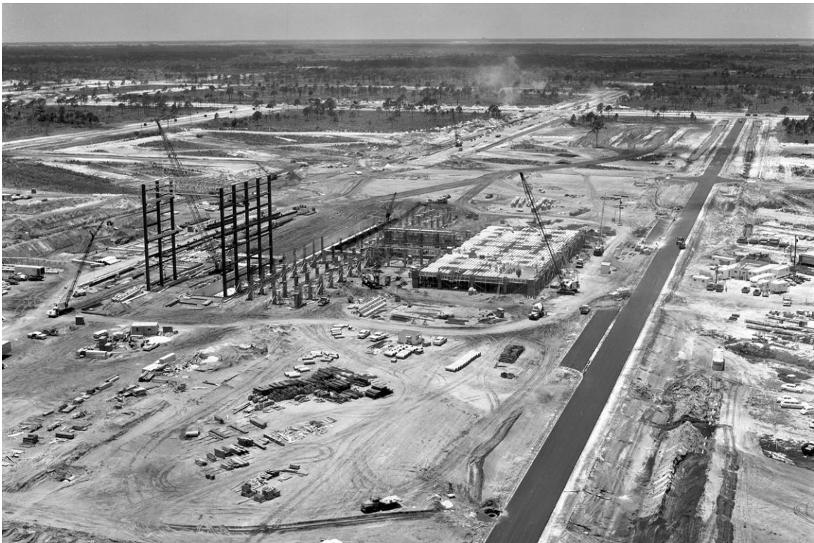
Figure B-3. Aerial showing early construction of O&C Building, facing southwest, June 4, 1963. Source: John F. Kennedy Space Center Archives, LOC-63-5667.
