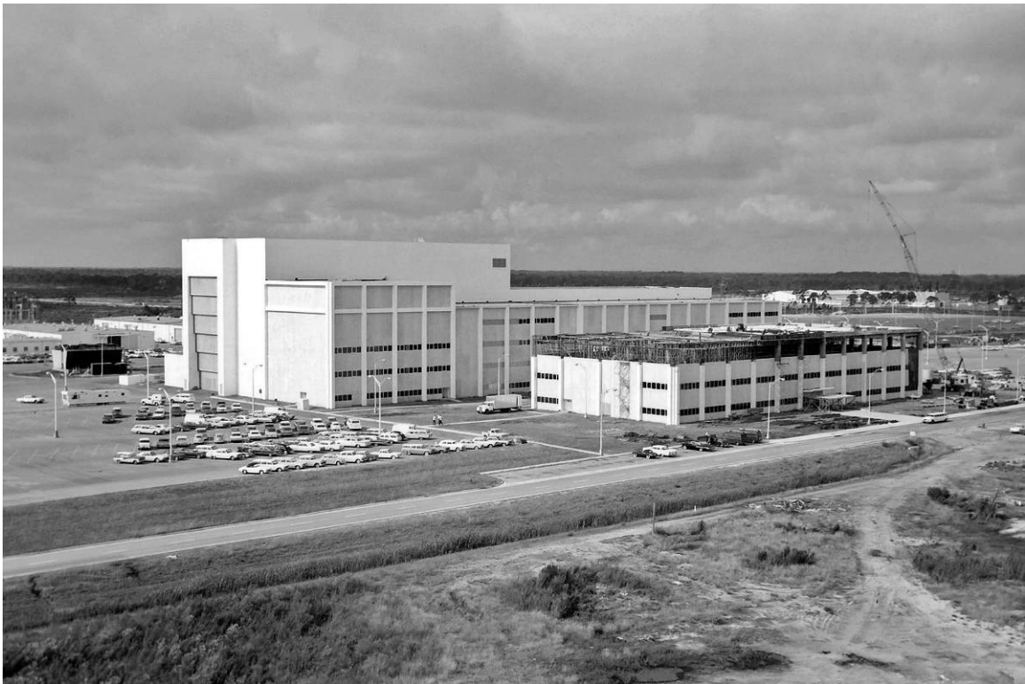
Figure B-8. Construction of the third floor of the O&C Building north wing, facing southwest, September 3, 1964.
