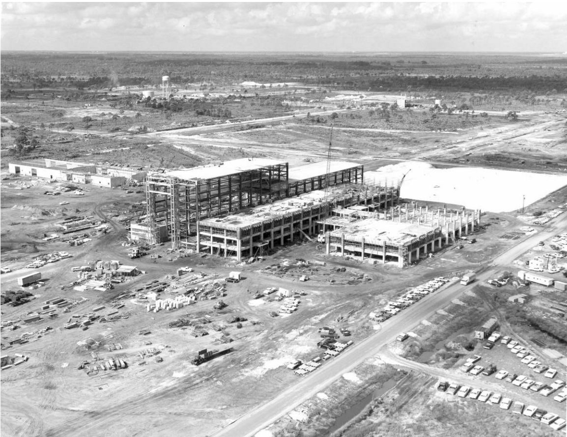
Figure B-5. Construction of the O&C Building, facing southwest, August 27, 1963. Source: John F. Kennedy Space Center Archives, LOC-63-8557.
