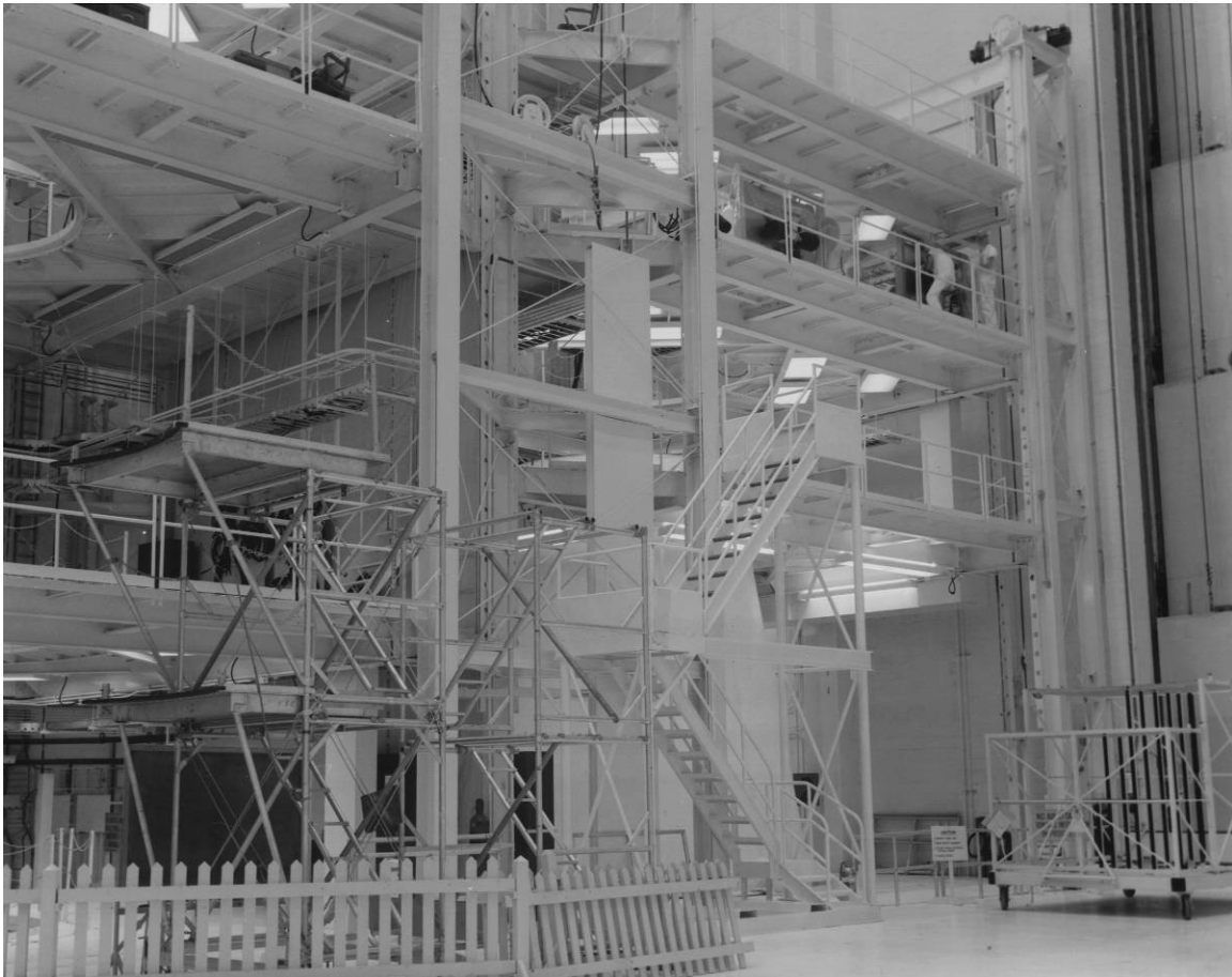
Figure B-12. Construction of the Lunar Module assembly and test area, facing northeast, August 15, 1966.
