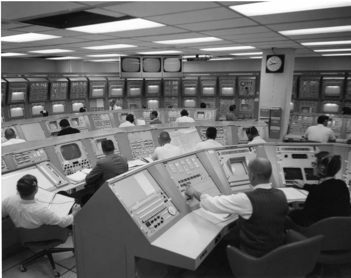
Figure B-17. View of Acceptance Checkout Equipment Station No. 1, direction unknown, February 16, 1967.
