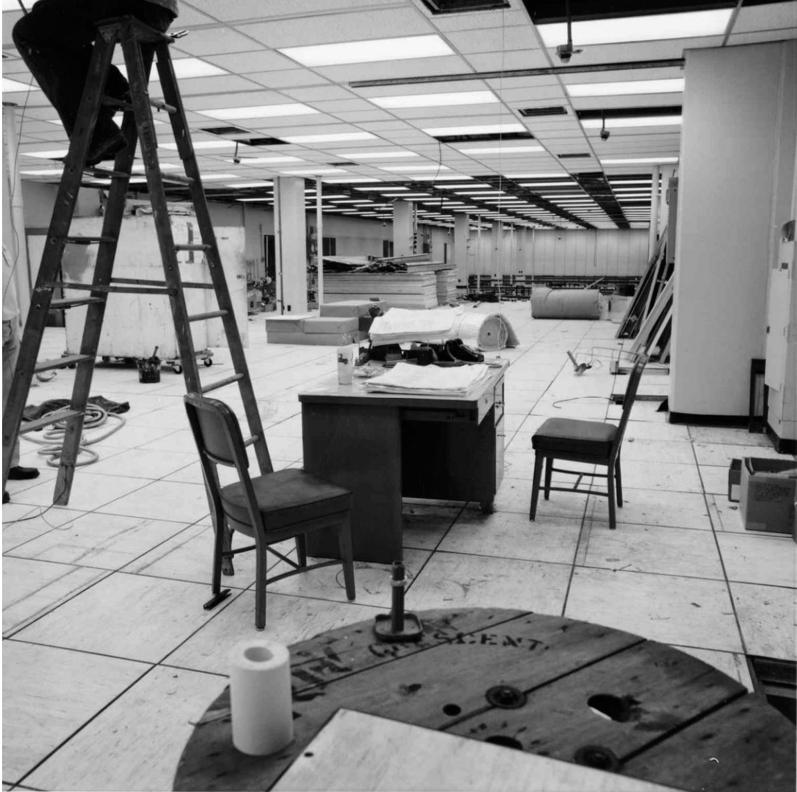
Figure B-18. Renovation of an Acceptance Checkout Equipment Station into Payload User Room Nos. A and B, direction unknown, April 28, 1981.
