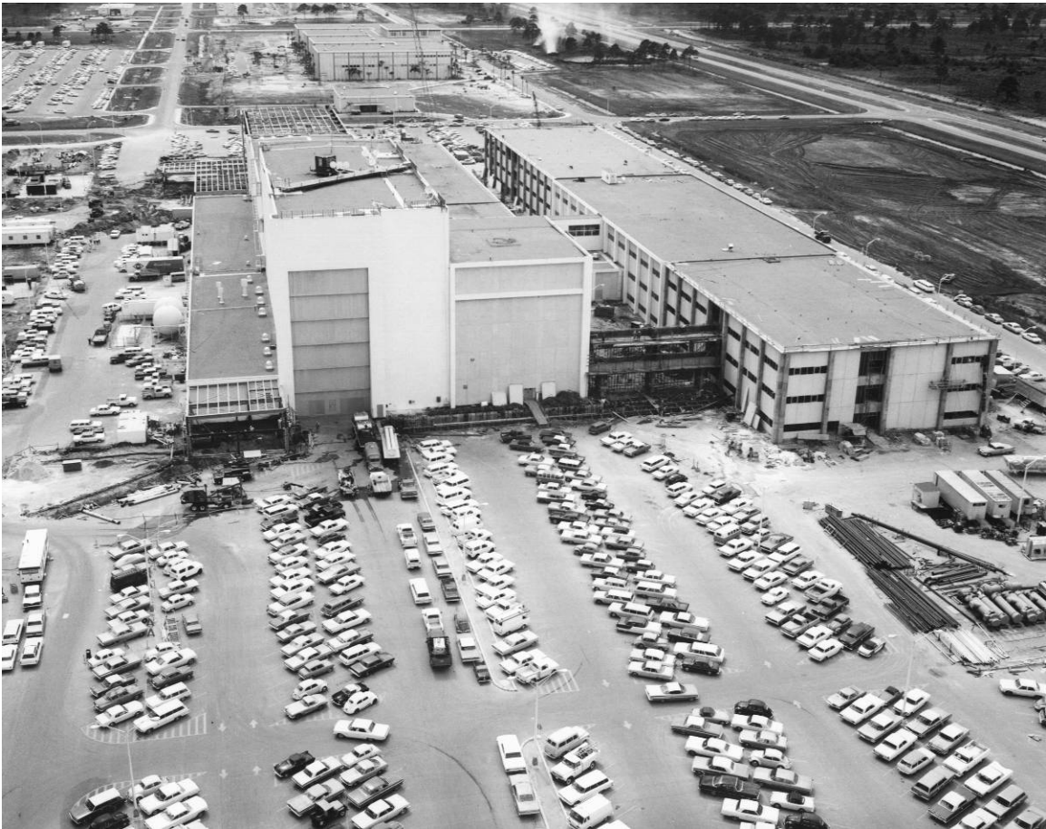
Figure B-9. Construction of the east and west additions to the O&C Building, facing west-northwest, August 5, 1965.
