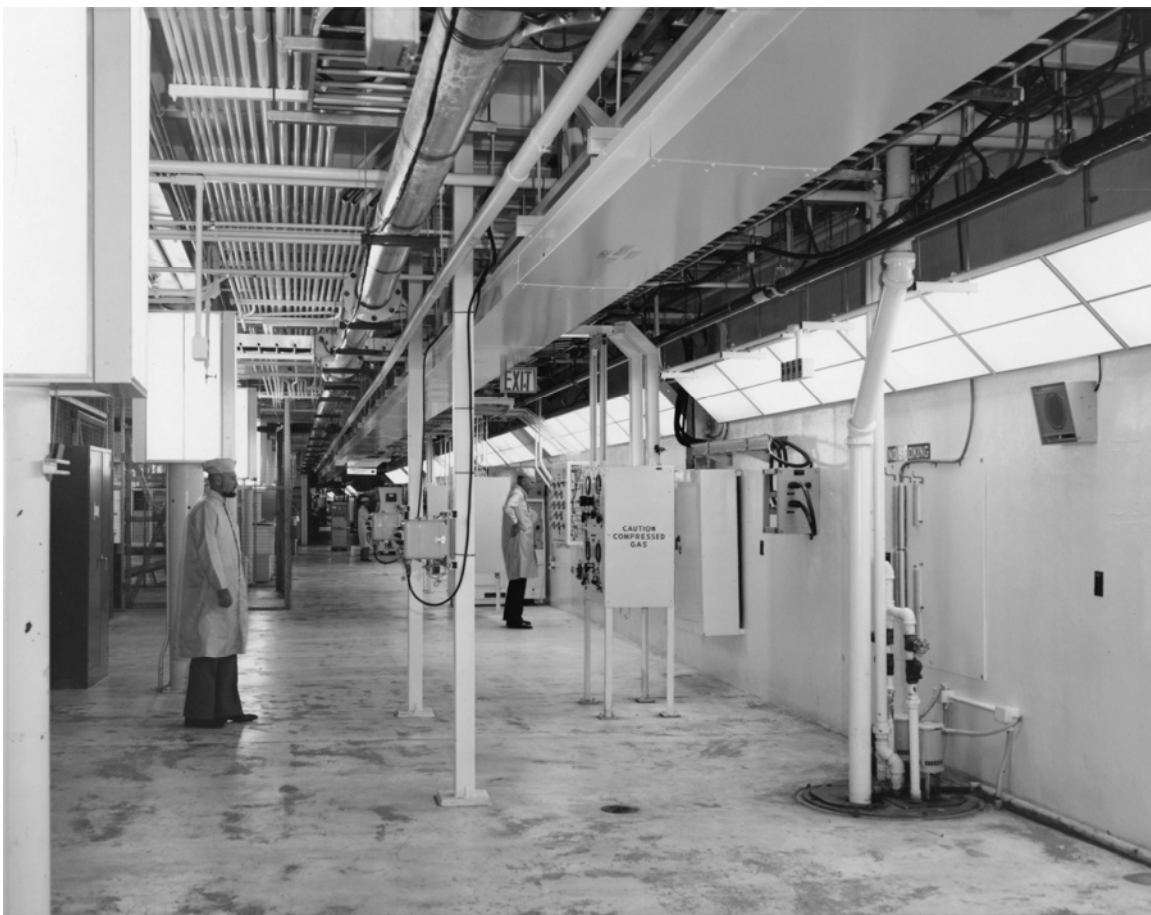
Figure B-27. View of the cable/utility tunnel, February 6, 1974. Source: John F. Kennedy Space Center Archives, 108-KSC-74C-82.
