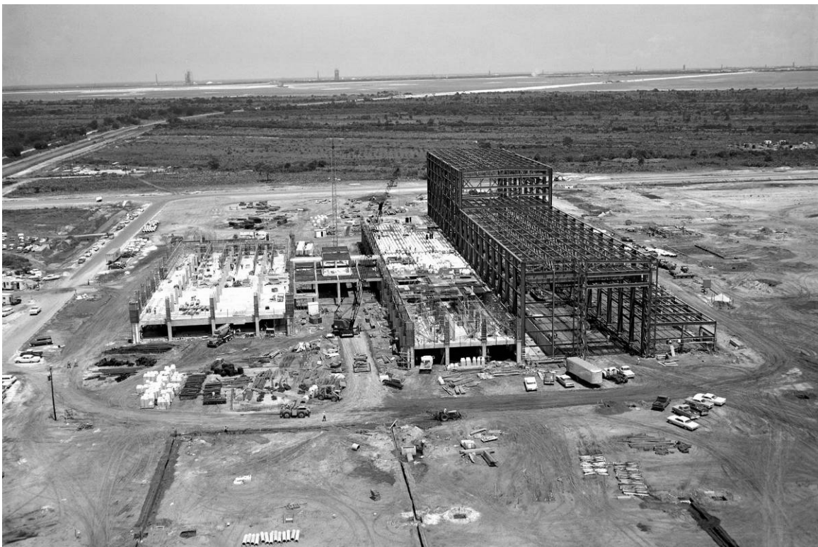
Figure B-4. Construction of the O&C Building, facing east, July 29, 1963. Source: Kennedy Institutional Imaging Facility, KSC-63C-2376.
