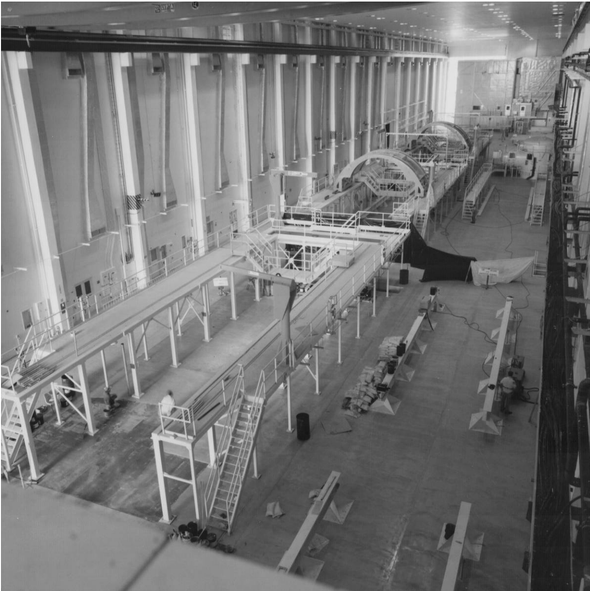
Figure B-16. Construction of the Spacelab workstands in the Low Bay, direction unknown, May 31, 1978.
