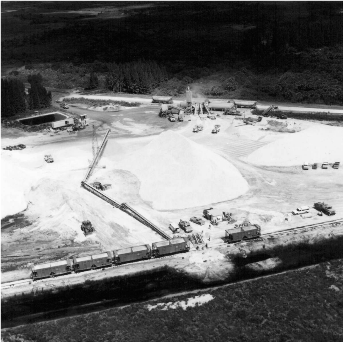
Figure A-7. Delivery of construction materials for the SLF runway via the railroad, August 4, 1975.
