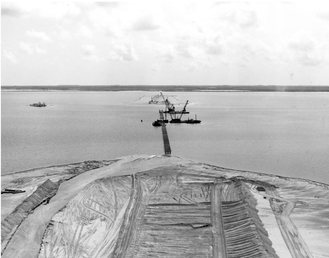
Figure A-4. Construction of the Jay Jay Bridge, 1963. Source: John F. Kennedy Space Center Archives, LOC-63-8518.
