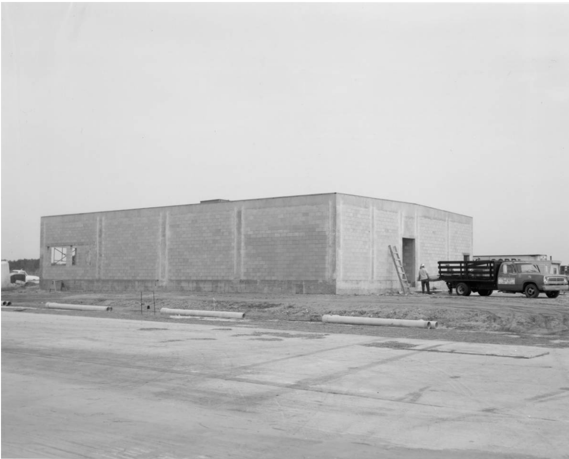
Figure A-9. Construction progress on LACB, camera facing northeast, January 16, 1976. Source: John F. Kennedy Space Center Archives, 108-KSC-76C-10005.
