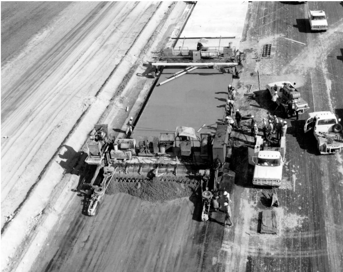
Figure A-4. Detail view of SLF showing concrete being poured, camera facing north, May 28, 1975.
