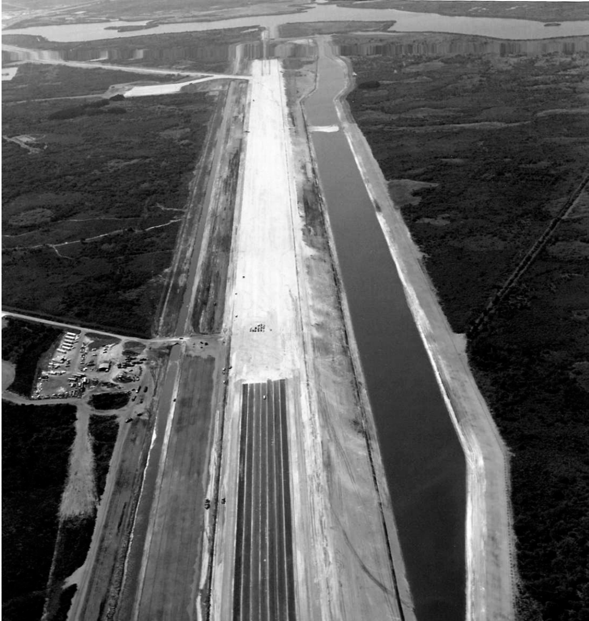
Figure A-3. View of SLF, showing construction progress, camera facing southeast, April 28, 1975.
