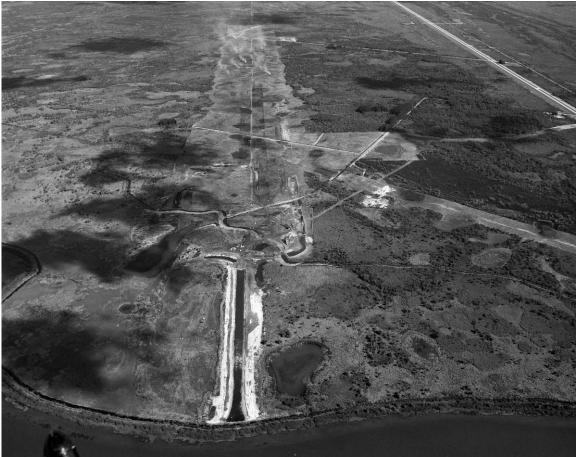
Figure A-2. View of SLF site, showing construction progress, camera facing north, October 9, 1974.
