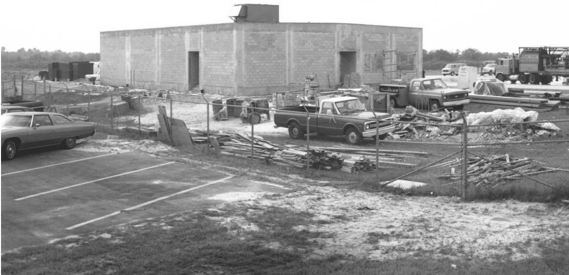
Figure A-8. Construction progress on LACB, camera facing southwest, January 16, 1976. Source: John F. Kennedy Space Center Archives, 108-KSC-76C-10006.
