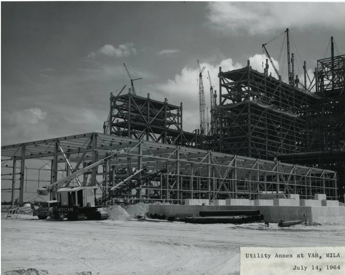
Figure B-1. Construction of the VAB Utility Annex, facing northeast, July 14, 1964. Source: John F. Kennedy Space Center Archives, 100-KSC-64-15109.
