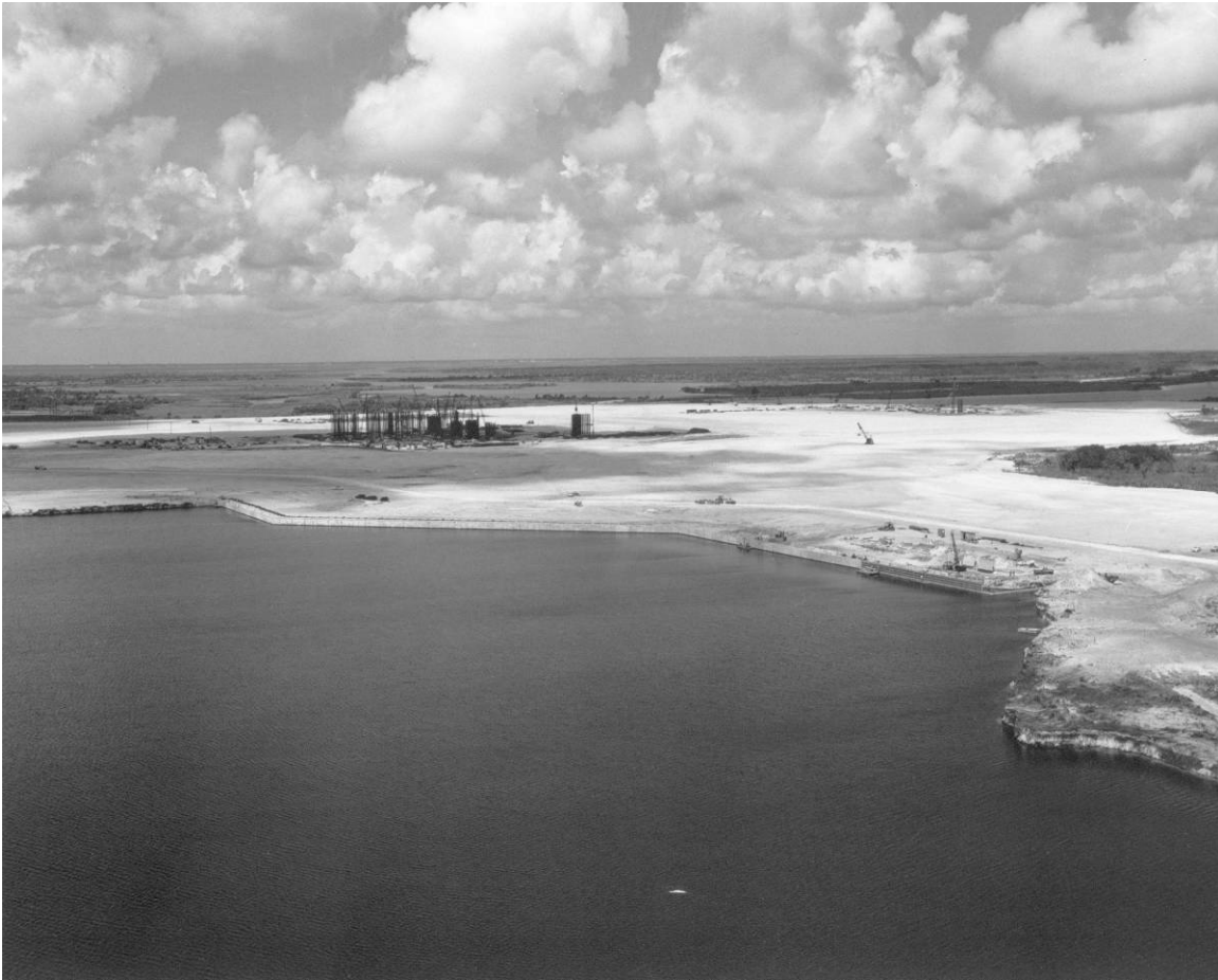
Figure D-7. View of the Barge Terminal Facility (early construction work on the VAB in the background), facing northwest, September 10, 1965.
