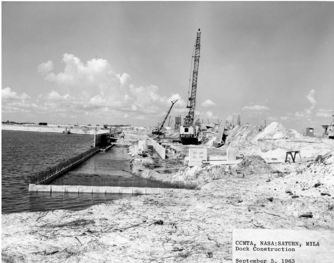
Figure D-6. Construction of the Barge Terminal Facility headwall and dock, facing southwest, September 5, 1963.
