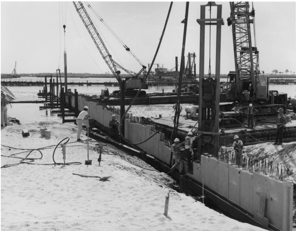
Figure D-4. Construction of the headwall, direction unknown, July 17, 1963. Source: John F. Kennedy Space Center Archives, LOC-63-7283.
