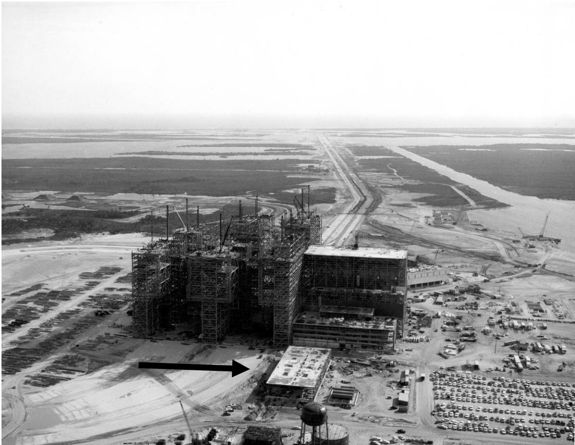
Figure B-2. Construction of the VAB and VAB Utility Annex (denoted by arrow), facing east, October 13, 1964.
