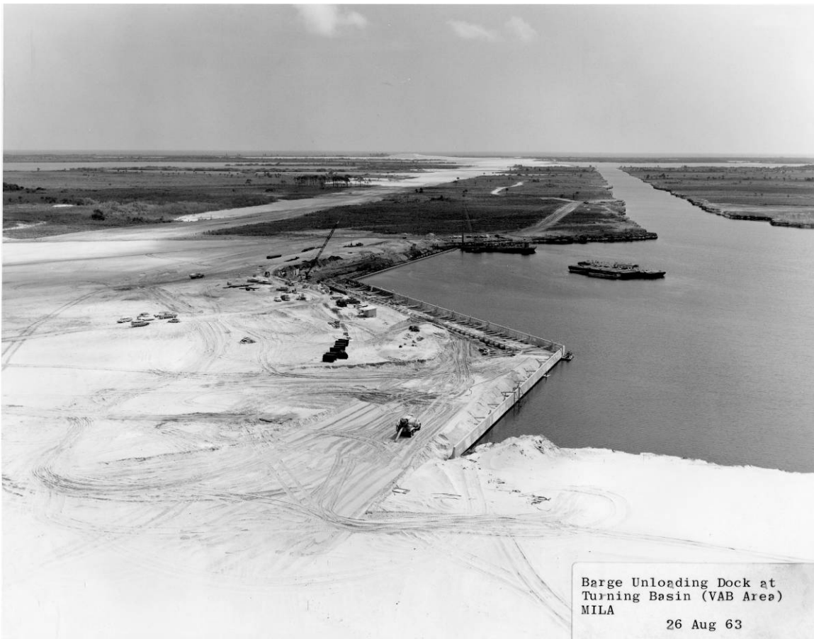
Figure D-5. Construction of the Barge Terminal Facility headwall and dock, facing northeast, August 26, 1963.
