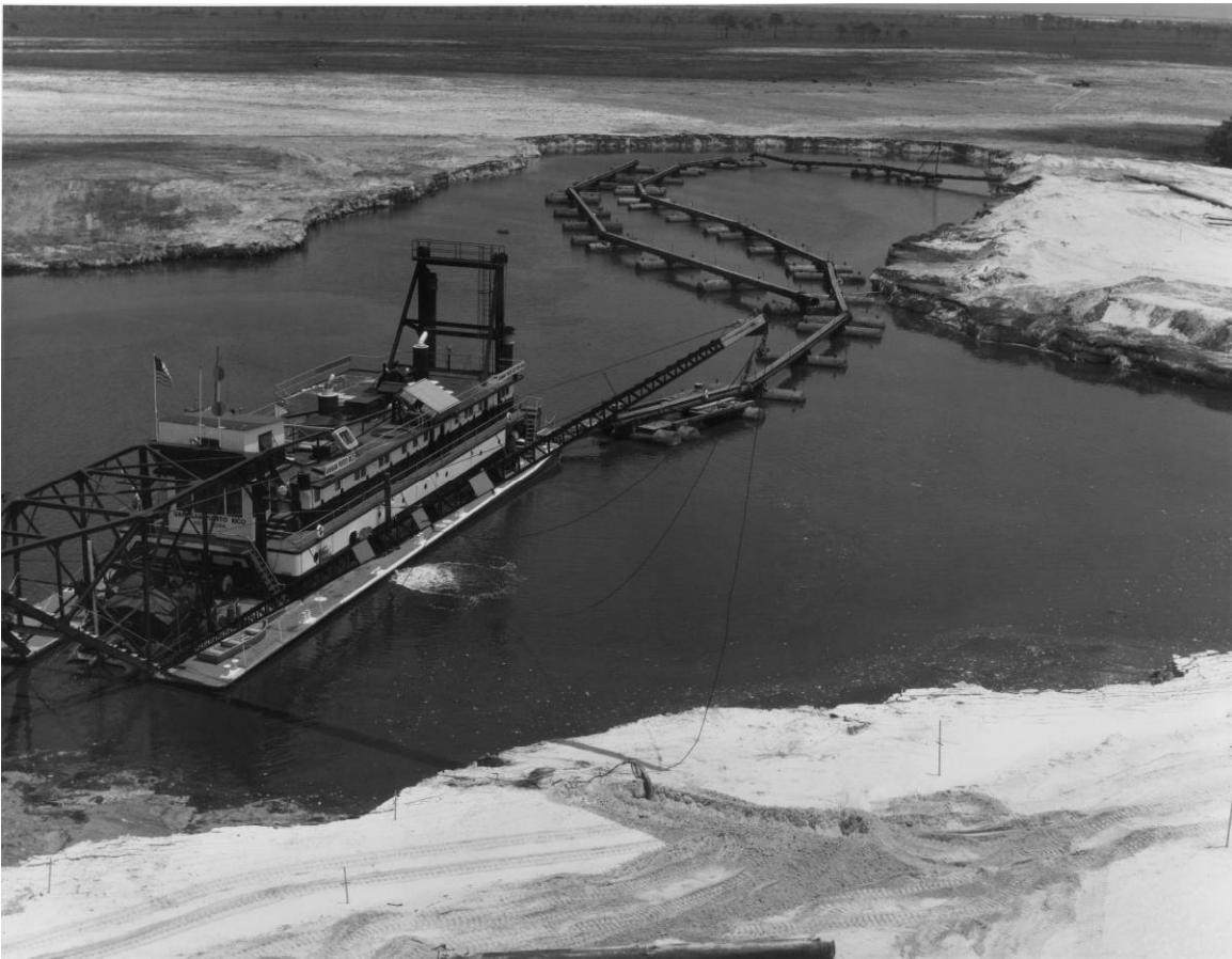
Figure D-2. Dredging of the Barge Terminal Facility, direction unknown, May 16, 1963. Source: John F. Kennedy Space Center Archives, LOC-63-5287.
