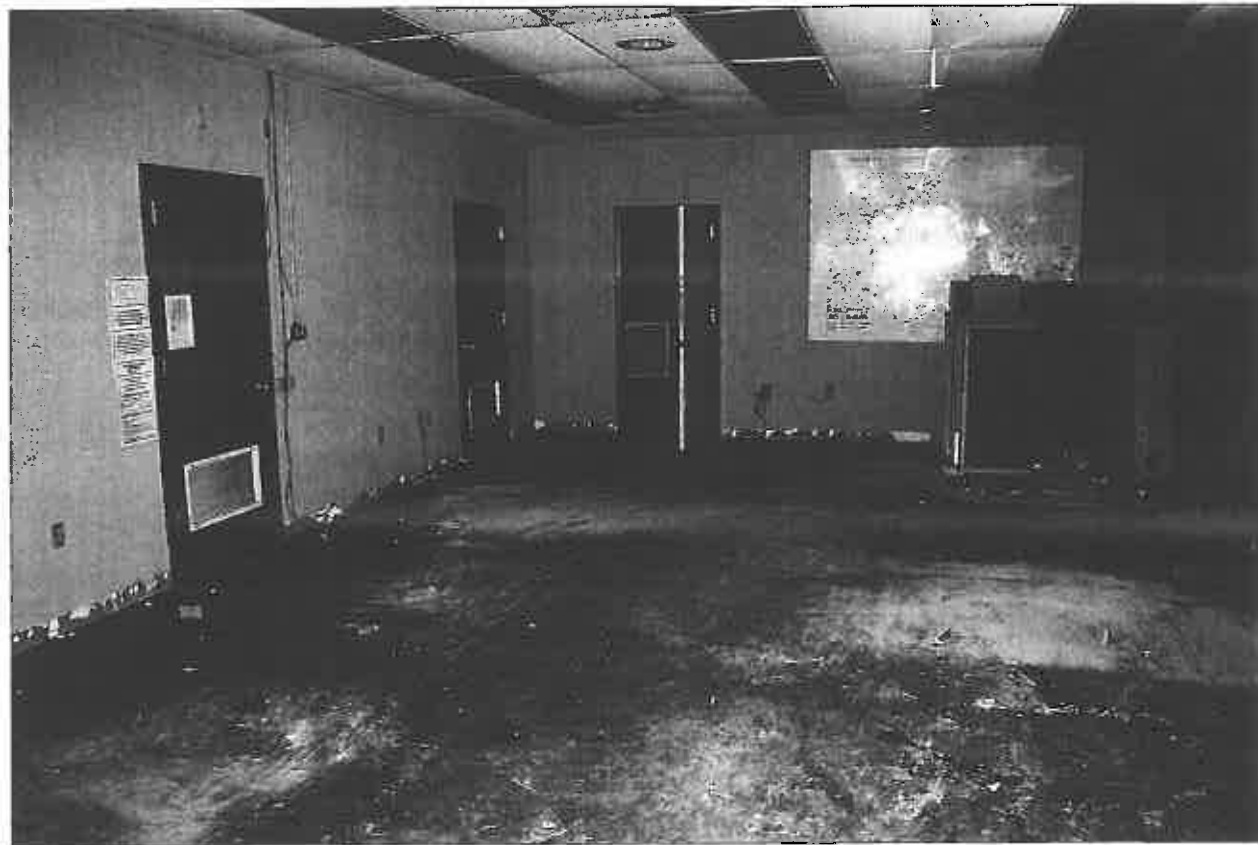
Hangar S, View of a Room in the Former Astronaut Quarters Area, View Southeast
