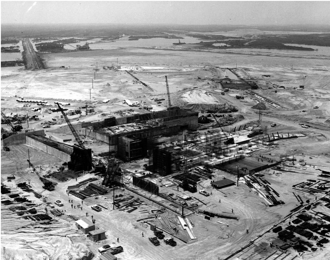
Photo B-2. Aerial view of LC39A hardstand construction, 1964. Source: John F. Kennedy Space Center, KSC-64C-2980, accessed via NIX at http://nix.nasa.gov/ .
