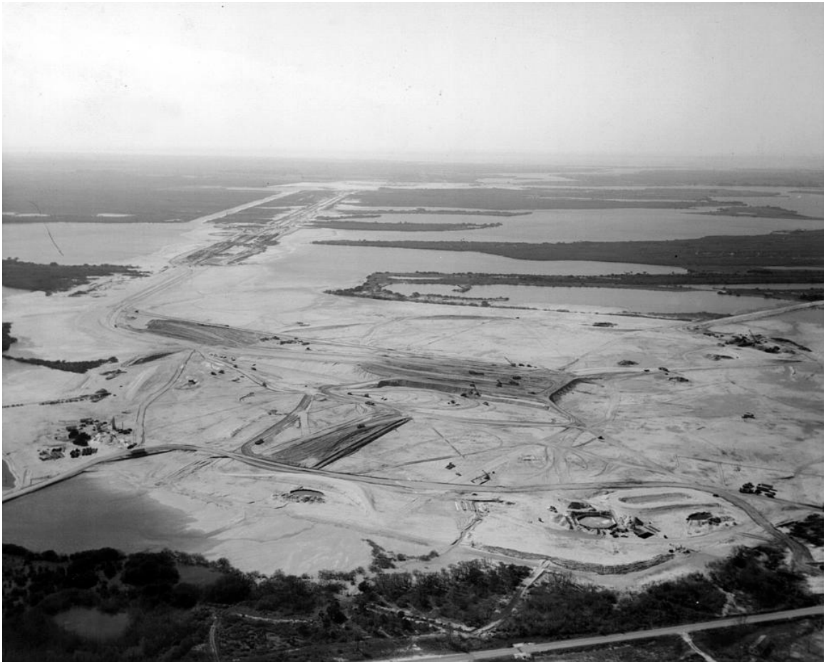
Photo B-1. Aerial view of Launch Complex 39A construction, January 14, 1964. Source: John F. Kennedy Space Center, KSC-64C-0027; accessed via NASA Image Exchange (NIX) at http://nix.nasa.gov/ .
