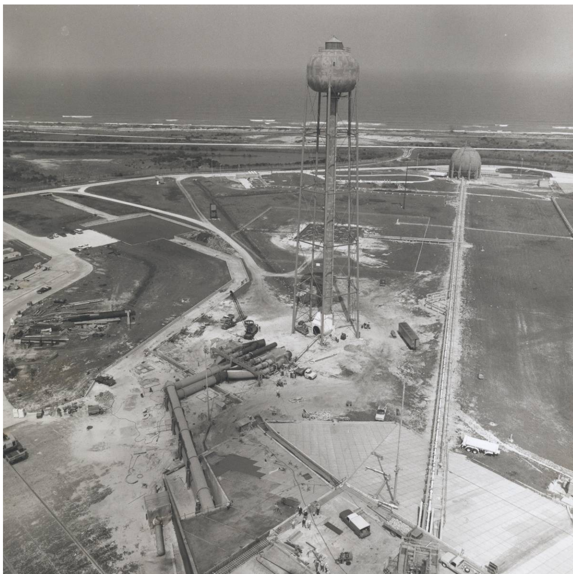
Photo B-10. Construction of the LC39A Sound Suppression System, March 28, 1978. Source: John F. Kennedy Space Center Archives, 108-KSC-378-298 Frame 4.
