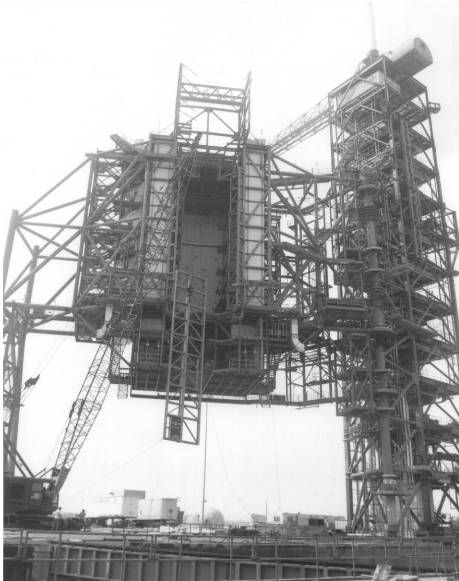
Photo B-8. Construction of the Payload Changeout Room at LC39A, September 9, 1977. Source: John F. Kennedy Space Center Archives, 108-KSC-77PC-311.
