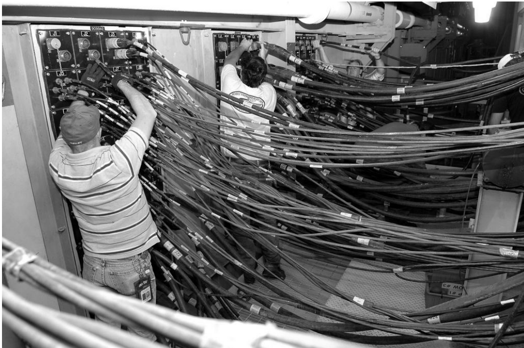
Figure A-9. Workers disconnect electrical and communications fittings between Mobile Launcher Platform and launch pad, May 7, 2004.
