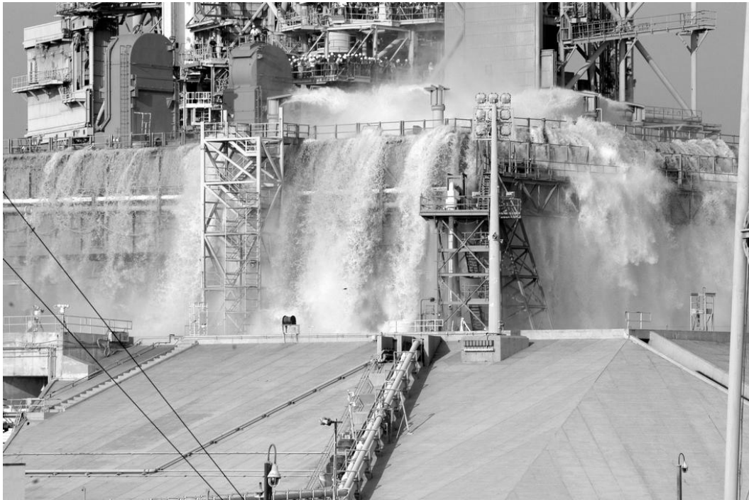
Figure A-8. Water sound suppression test at launch pad, note water coming out of spray pipes, May 7, 2004.
