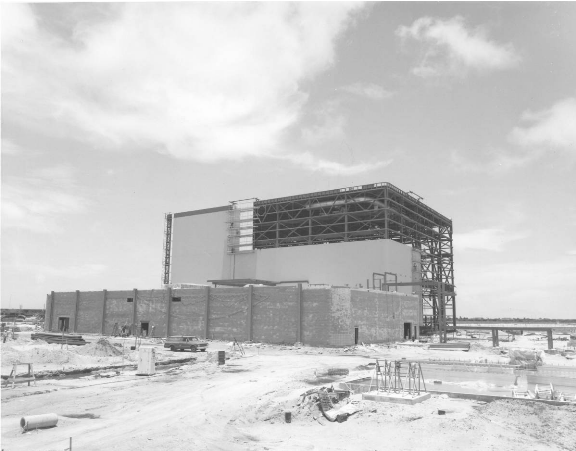
Figure B-1. View of OPF High Bay No. 1 and Low Bay construction, 1976. Source: John F. Kennedy Space Center Archives, 108-KSC-76-1545.
