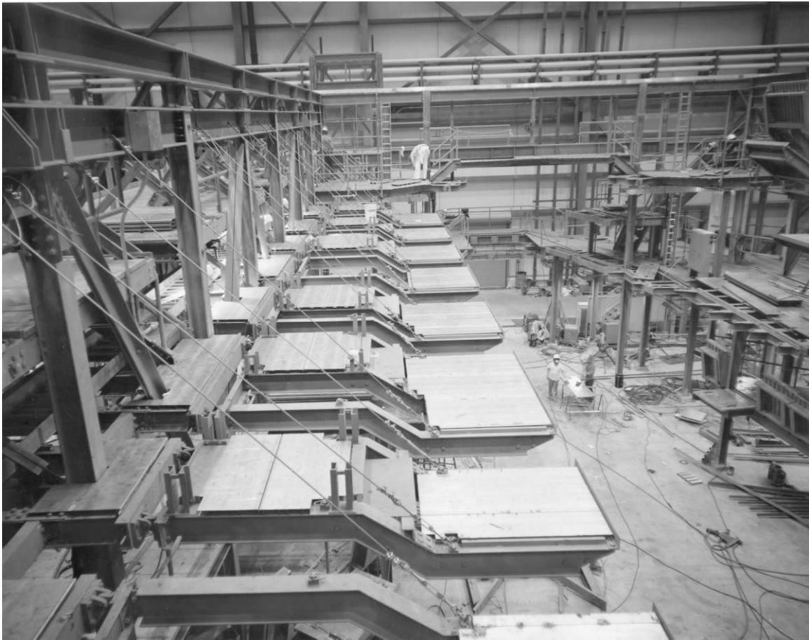
Figure B-5. View of OPF High Bay No. 1, Level 13 platform installation, July 8, 1977. Source: John F. Kennedy Space Center Archives, 108-KSC-77C-1228.
