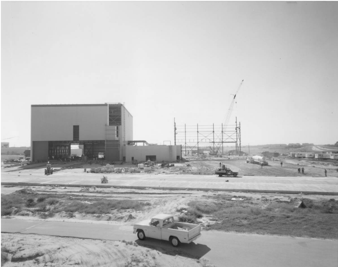
Figure B-3. View of OPF High Bay No. 2 construction, 1976. Source: John F. Kennedy Space Center Archives, 108-KSC-76-2986.
