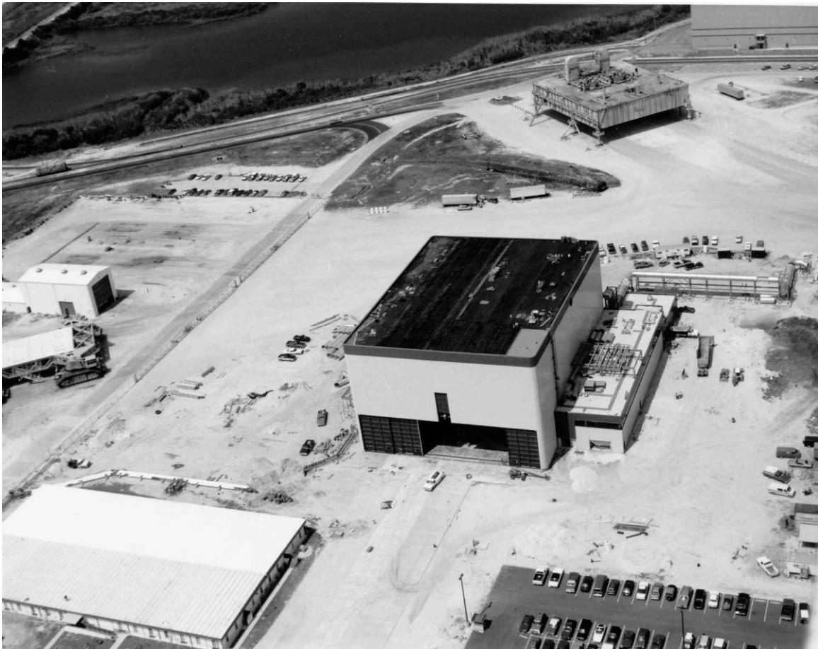
Figure A-1. Aerial view of OPF-3 construction, March 17, 1987. Source: John F. Kennedy Space Center Archives, KSC-387C-565-7.
