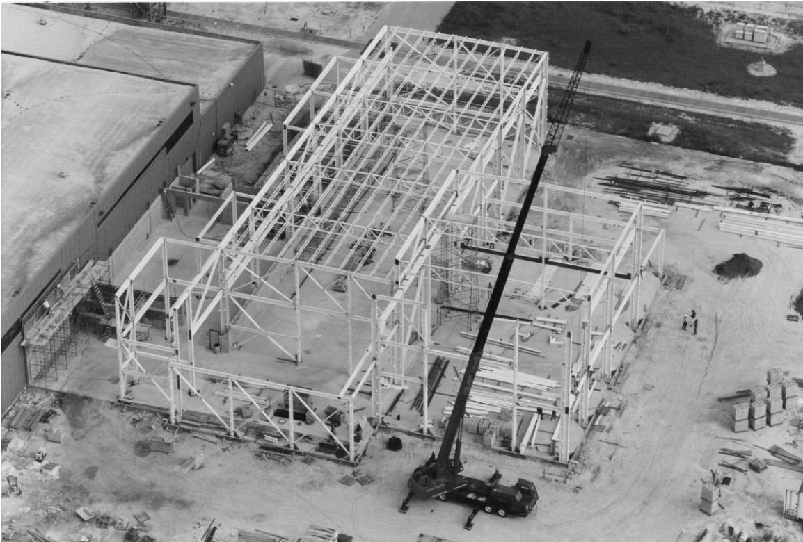
Figure A-3. Detail view of SSMEPF construction, May 23, 1997. Source: John F. Kennedy Space Center Archives, KSC-97PC-835.
